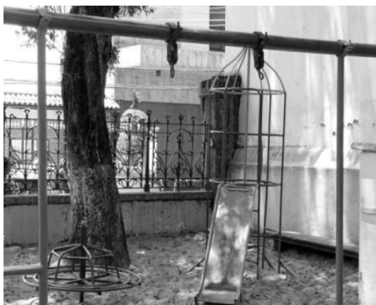
Figure 45- Slide with a worn off paint in School 3
