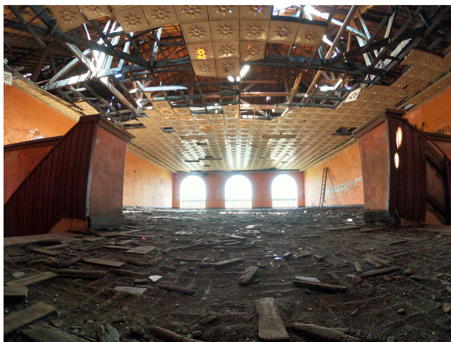
FIGURE 13 Great hall on the upper level, above the foyer. Source: Janaína da Silva Alves, September/2021, private archive.
