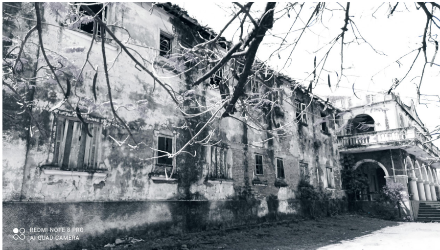
FIGURE 5 Left lateral of the hotels' façade. Degradation and time action in windows and walls can be observed. Source: Janaína da Silva Alves, September/2021, private archive.
