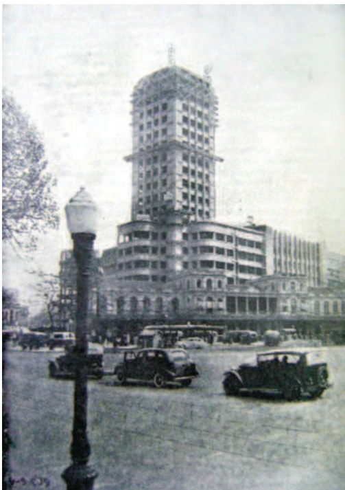
Picture 4: view of D. Pedro II Station under construction, overlooking the old Campo Station, demolished in 1940 after the completion of the works. Source: Civil Service Magazine , Jul. -Aug. 1939, p. 70.
